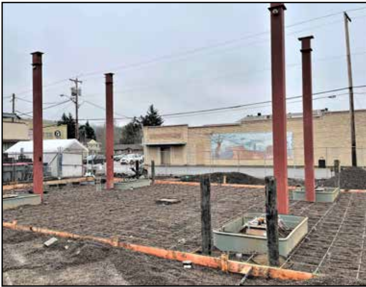
The new gas station under construction on the corner of West Main and North Bridge is all set for a concrete pour.
