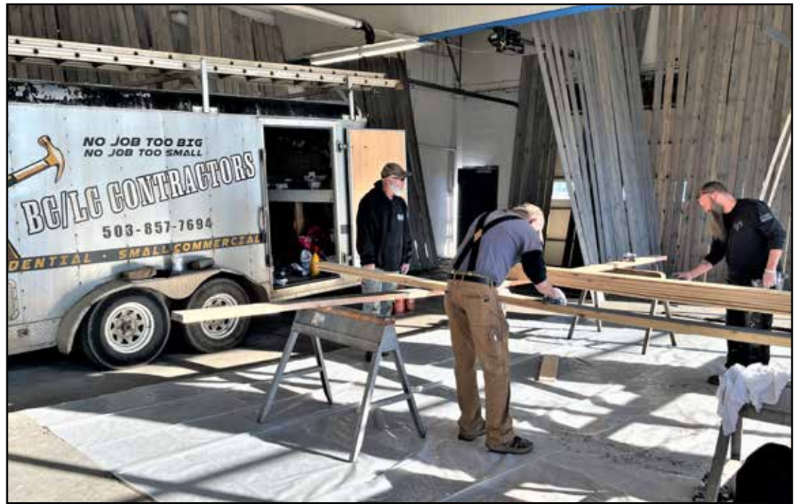
BC/LC Contractors crew, working in the former Terry's Auto Repair shop at 131 SE Sheridan Road, is prepping the wood to be used for the new ceiling they will install at TJ's Superette, 129 W. Main Street. The BC/LC crew said the company is looking into renting the space to use for their shop.
