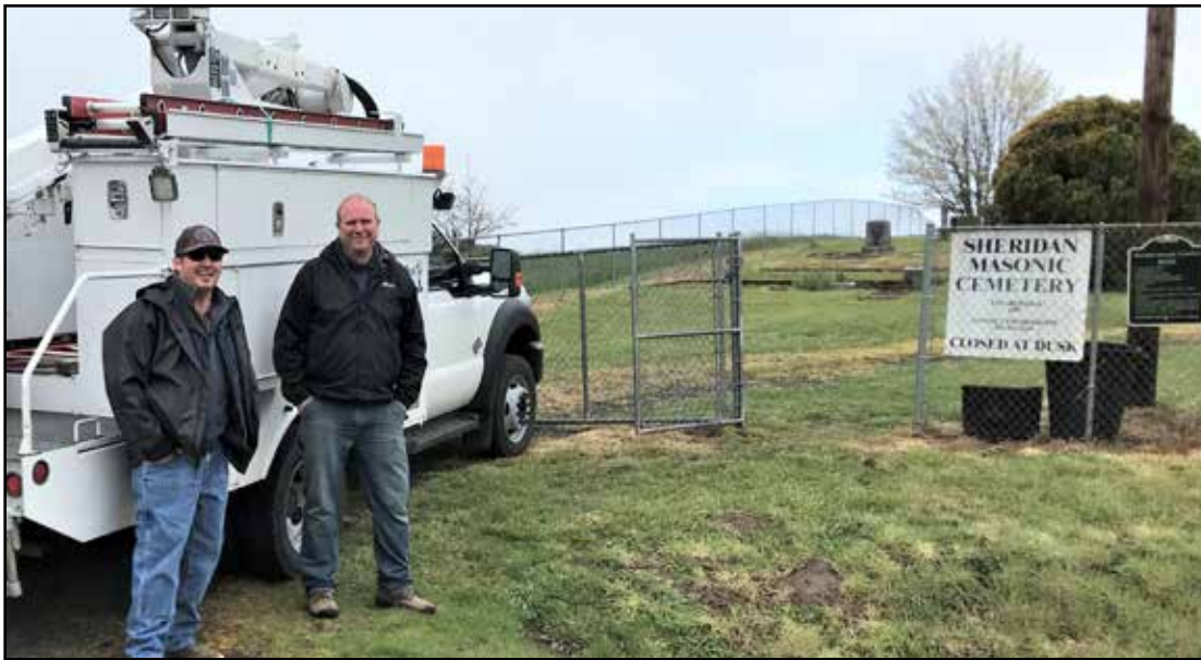
Special thanks to Aaron and Melissa Clemmer at Stuck Electric for sending Marcus Cox and Erik Rogers out to repair lights that were not working at the Masonic Cemetery in Sheridan. Marcus updated both lights with new LED bulbs and added new photo eyes. Great job, guys! (Photo and information courtesy of Mike Spencer.)
