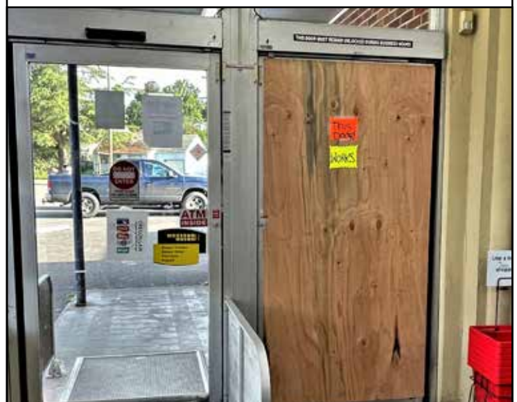
Thieves who broke into the Willamina IGA last week broke glass and damaged both front entryways. They managed to steal 10 packs of cigarettes.
