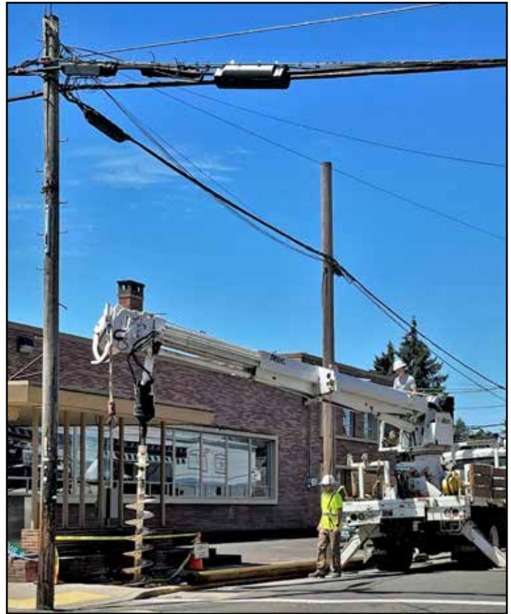
Joseph with C-2 Utility Contractors, LLC, of Coburg, Ore., said the pole on the corner of South Bridge and Monroe (next to U.S. Bank) needed to be replaced. The old pole was removed, a new pole installed, and the old wiring was moved to the new pole. C-2 is a utility contractor for Century Link, who owns this pole.
