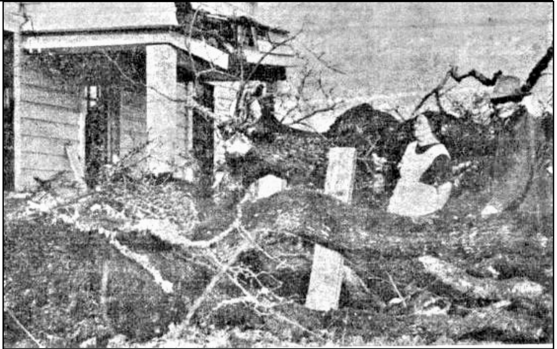
PORCH ON THE HOME of Mr. and Mrs. D.E. Blanchard in the Harmony district southwest of Sheridan was damaged as well as the roof of the house in the severe wind storm early Thursday morning, January 7. Pictured above are Mr. and Mrs. Blanchard surveying the damage to the home when a huge oak tree, five-feet in diameter split and came crashing down on the porch. Damage was caused about 4 a.m. The Blanchard home is one of the older houses in the area being built more than 80 years ago. Mr. and Mrs. Blanchard bought the farm six years ago. It is known as the John Guttry farm. Mr. Blanchard worked on the farm many years and always had a strong desire to be its owner.
