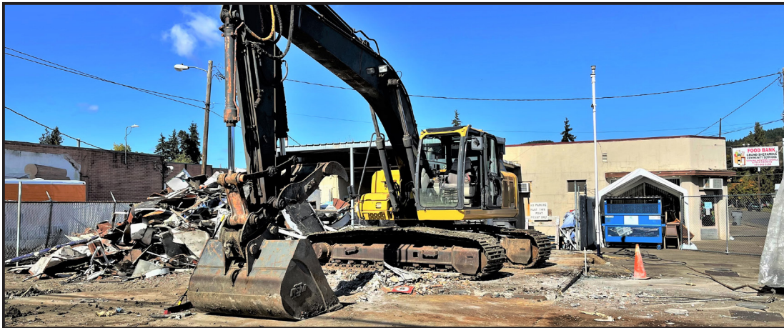
Central Service Inc., an Oregon-based company that specializes in all aspects of petroleum construction, tackled the demolition in full force on Wednesday and Thursday, Oct. 6 and 7.
