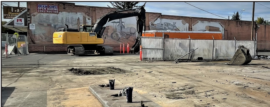
By Friday, Oct. 8, the shop building and pumps were removed and the debris had been hauled away.
