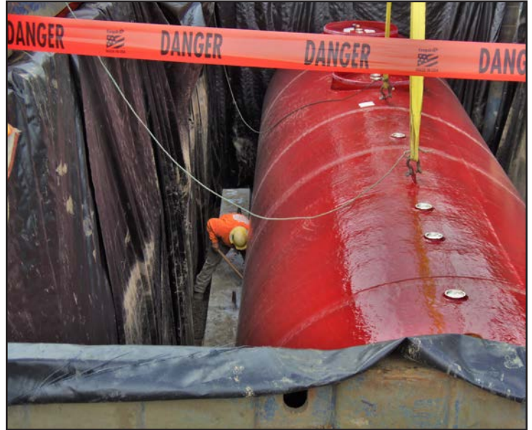
placement of the new fuel tank shown right. The fuel tank has separate compartments inside that will allow this one tank to hold diesel and different grades of gasoline.
