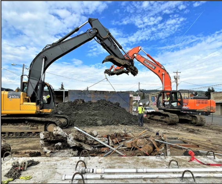
The reconstruction of TJ's Gas Station, 107 W. Main Street in Sheridan, has continued to make tremendous strides over the past week. The photo on the left shows two excavators preparing for
