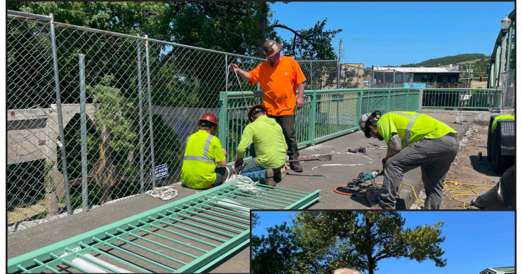
Yamhill County workers partnered with City of Sheridan to install the new railings in front of where the old Masonic Lodge stood until its collapse in January of 2021.
