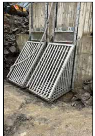
The city's new water intake system designed to require less interaction for maintenance purposes.
