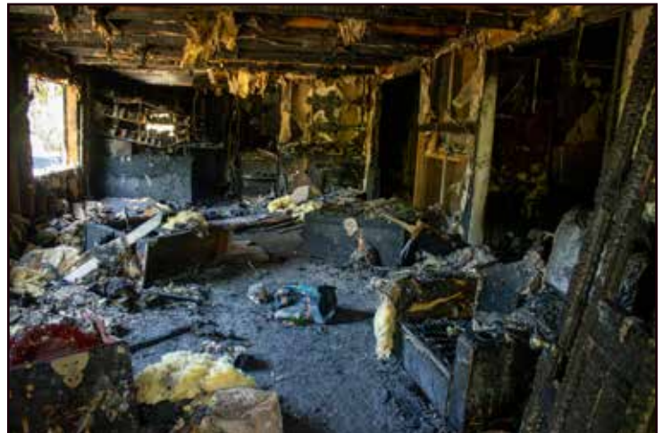
The aftermath of a fire that burned through this house the evening of July 4. The fire got hot enough to melt the refrigerator.
