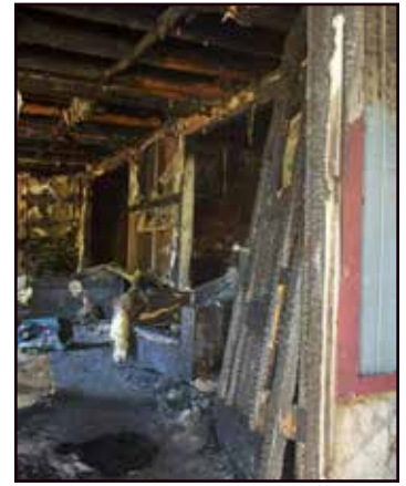
The remains of the door used by the family to exit the fire-engulfed building last Friday.
