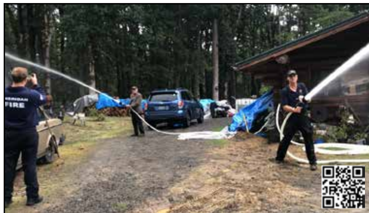
Rich Hoffmann (right) demonstrates his exterior fire protection system, using two fire attack hose lines to spray water and Class A wildland firefighting foam around a structure. The system is designed to provide immediate fire protection over a large area without waiting for a fire engine to arrive.
